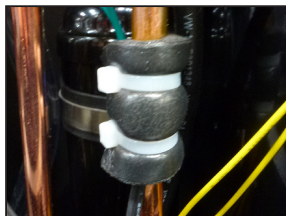
Figure 6: Thermistor attached to the refrigerant line.
